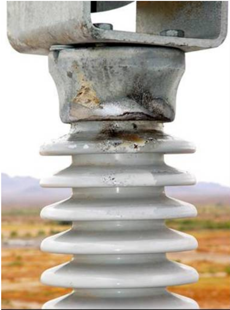
Fig. 2: Flashed 230 kV porcelain station post. Contamination was suspected as the root cause, but as is clear from the photograph, the insulator looks fairly clean.
