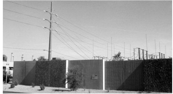
Fig. 2 Substation in Tempe, AZ
