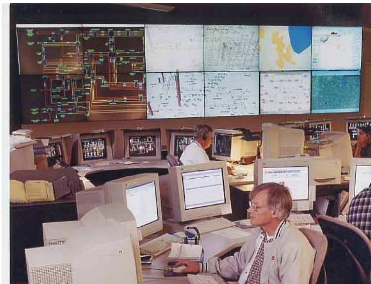
Figure 6: Commonwealth Edison Control Center in Northern Illinois. Control centers are busy places, with data coming from hundreds of sources that has to be quickly processed and interpreted. Visualization tools contribute to turning data into “information” useful for decision-making.
