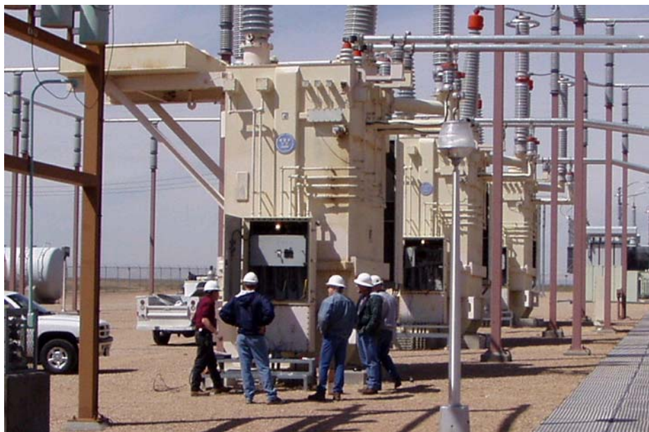
Figure 4.11: Three single-phase 166 MVA transformers used in experiment
