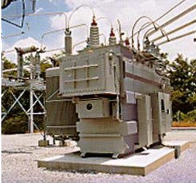
Figure 1.1: Typical large substation transformer
